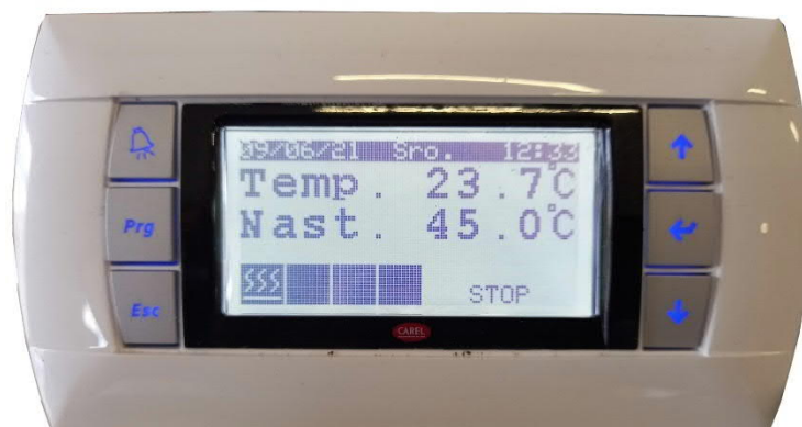
Rys. Terminal Carel
